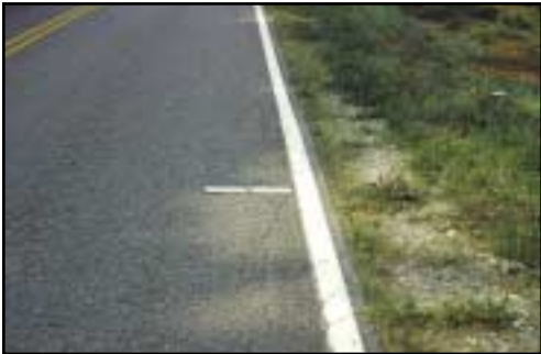
FIGURE 12 Distress Type ACP 3—Low Severity Edge Cracking
