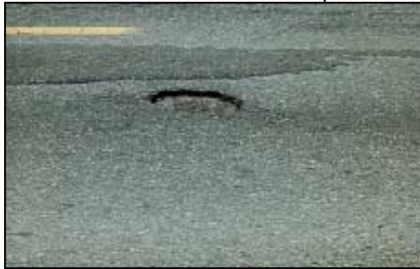
FIGURE 28 Distress Type ACP 8—Moderate Severity Pothole
