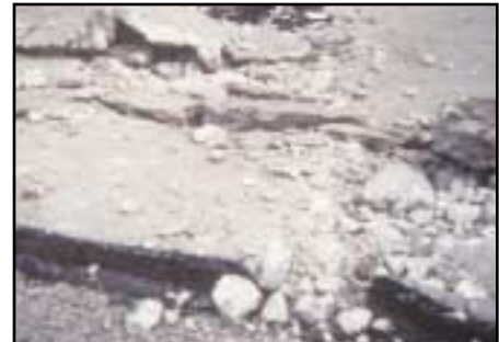
FIGURE 108 Distress Type CRCP 7—Close-up View of a Blowup
