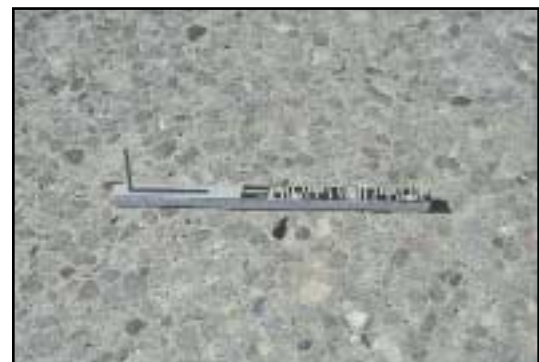
FIGURE 74 Distress Type JCP 10—A Popout
