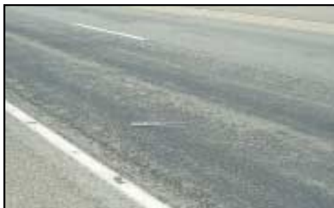
FIGURE 37 Distress Type ACP 11—Loss of Texture
