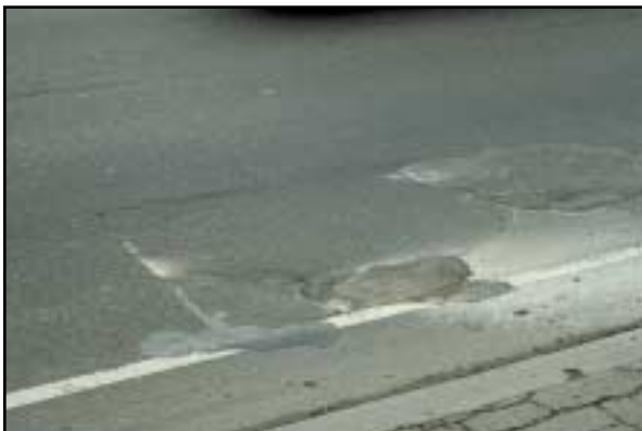
FIGURE 25 Distress Type ACP 7—High Severity Patch
