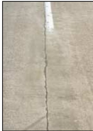
FIGURE 129 Distress Type CRCP 13—Low Severity Spalling of a Longitudinal Joint
