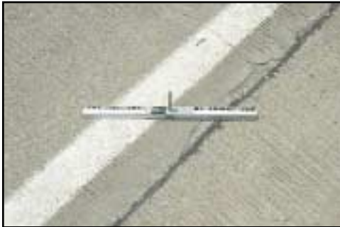
FIGURE 128 Distress Type CRCP 13—Close-up View of Low Severity Spalling of a Longitudinal Joint
