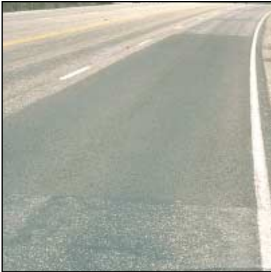
FIGURE 23 Distress Type ACP 7—Low Severity Patch
