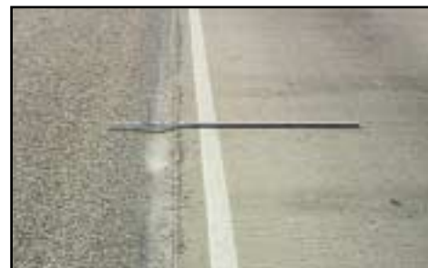
FIGURE 115 Distress Type CRCP 9—Lane-to-Shoulder Dropoff
