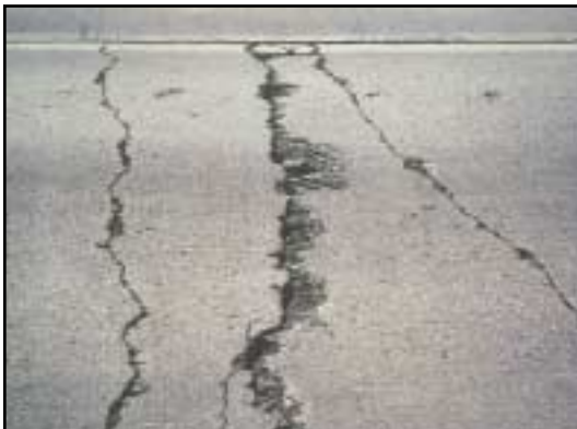
FIGURE 100 Distress Type CRCP 3—High Severity Transverse Cracking
