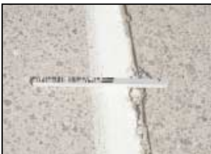
FIGURE 64 Distress Type JCP 6—Low Severity Spalling of Longitudinal Joint
