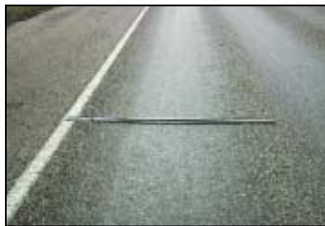
FIGURE 32 Distress Type ACP 9—Rutting
