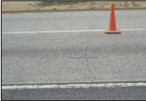
FIGURE 98 Distress Type CRCP 3—Low Severity Transverse Cracking
