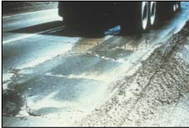
FIGURE 89 Distress Type JCP 16—Water Bleeding and Pumping
