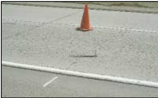
FIGURE 59 Distress Type JCP 4—Moderate Severity Transverse Cracking
