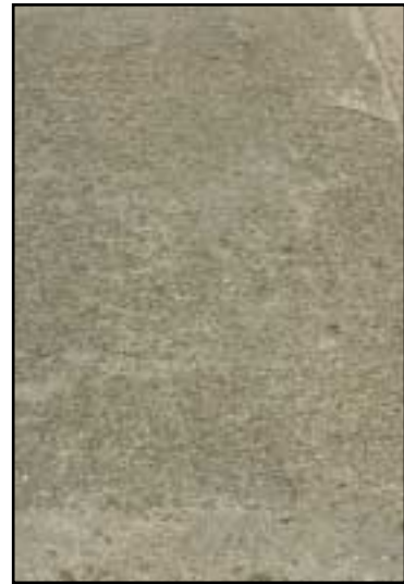
FIGURE 102 Distress Type CRCP 4b—Scaling
