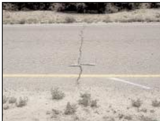
FIGURE 21 Distress Type ACP 6—High Severity Transverse Cracking
