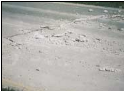
FIGURE 107 Distress Type CRCP 7—A Blowup
