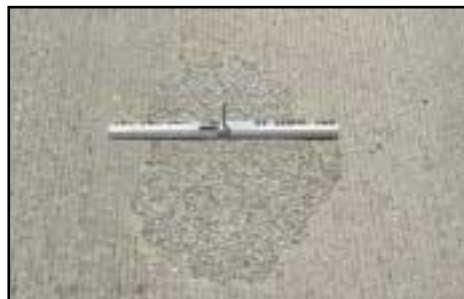
FIGURE 119 Distress Type CRCP 11—Small, Low Severity Asphalt Concrete Patch
