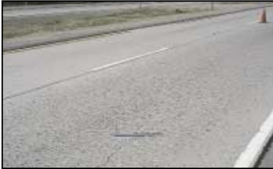
FIGURE 55 Distress Type JCP 3—Low Severity Longitudinal Cracking
