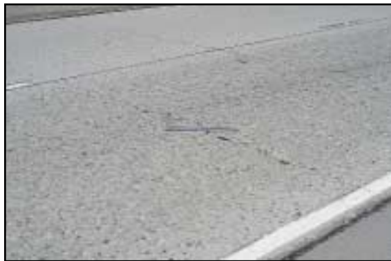
FIGURE 60 Distress Type JCP 4—High Severity Transverse Cracking
