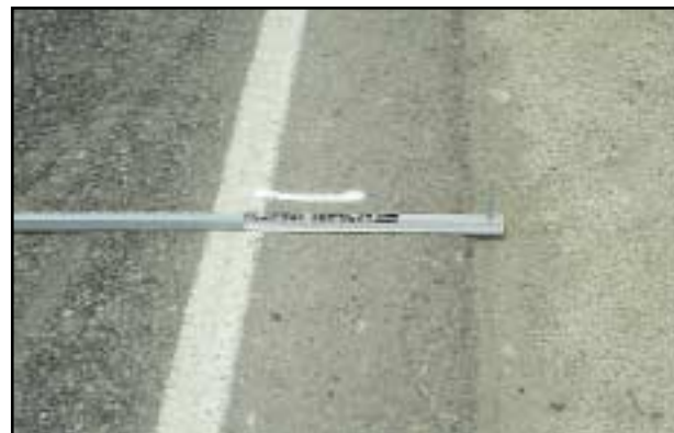
FIGURE 44 Distress Type ACP 14—Lane-to-Shoulder Dropoff
