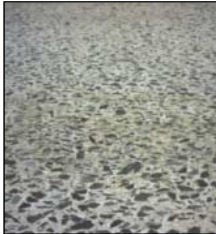
FIGURE 103 Distress Type CRCP 5—Polished Aggregate
