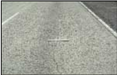
Figure 94 Distress Type CRCP 2—Low Severity Longitudinal Cracking
