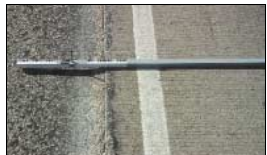
FIGURE 80 Distress Type JCP 13— Lane-to-Shoulder Dropoff
