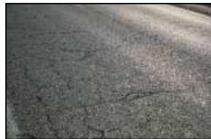
FIGURE 10 Distress Type ACP 2—High Severity Block Cracking
