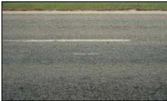
FIGURE 36 Distress Type ACP 11—Discoloration
