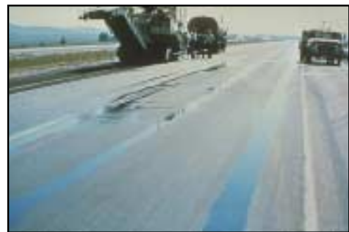
FIGURE 33 Distress Type ACP 9—Standing Water in Ruts
