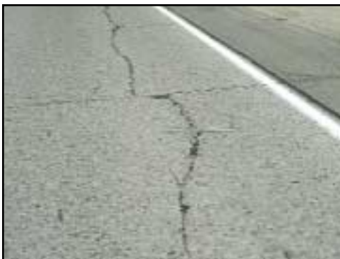
FIGURE 57 Distress Type JCP 3—High Severity Longitudinal Cracking
