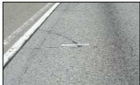
FIGURE 50 Distress Type JCP 1—Moderate Severity Corner Break
