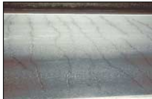
FIGURE 97 Distress Type CRCP 3—Transverse Cracking Pattern
