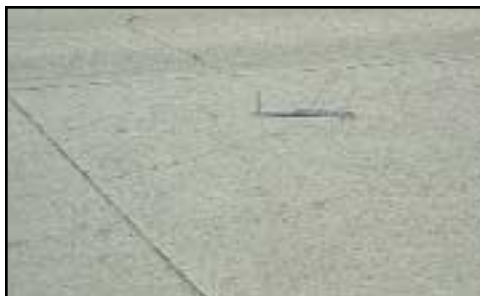
FIGURE 49 Distress Type JCP 1—Low Severity Corner Break
