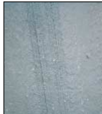
FIGURE 38 Distress Type ACP 11— Aggregate Obscured
