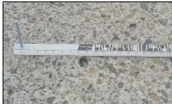
FIGURE 105 Distress Type CRCP 6—Popouts
