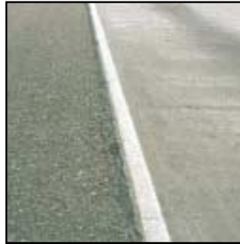
FIGURE 83 Distress Type JCP 14—Well-Sealed Lane-to-Shoulder Separation
