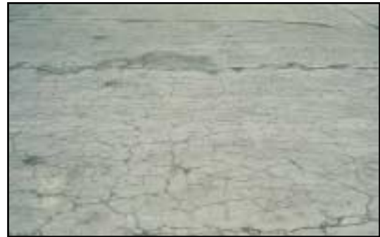
FIGURE 69 Distress Type JCP 8a—Map Cracking
