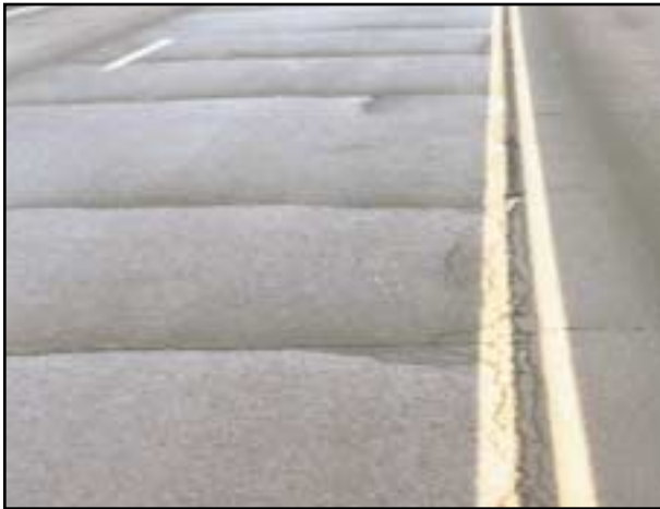
FIGURE 17 Distress Type ACP 5—High Severity Reflection Cracking at Joints
