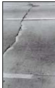
FIGURE 78 Distress Type JCP 12—Faulting of Transverse Cracks
