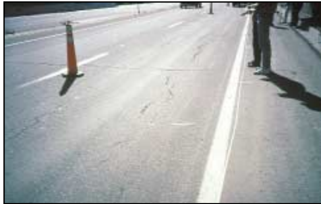
FIGURE 5 Distress Type ACP 1—Low Severity Fatigue Cracking
