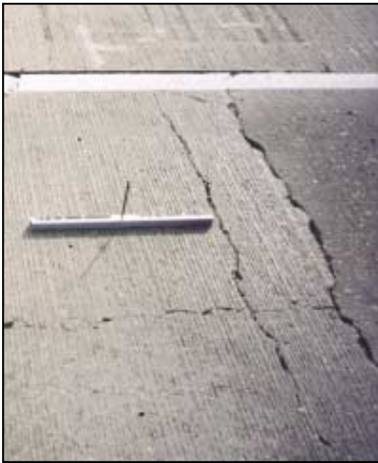
FIGURE 125 Distress Type CRCP 12—Moderate Severity Punchout
