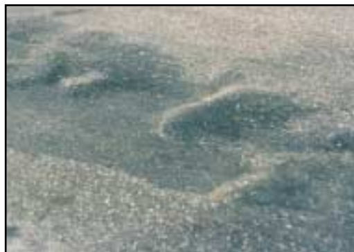
FIGURE 35 Distress Type ACP 10—Shoving in Pavement Surface
