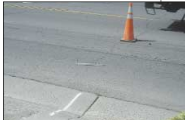
FIGURE 20 Distress Type ACP 6—Moderate Severity Transverse Cracking
